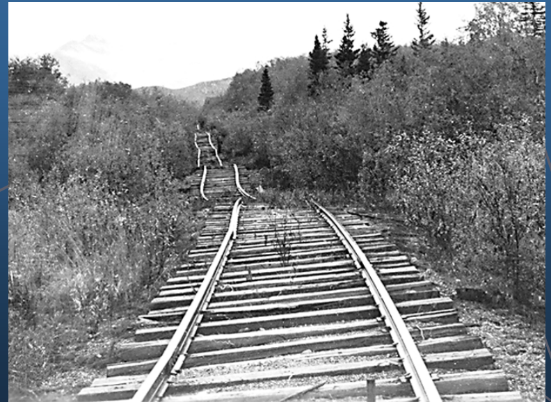
Damage due to thermal permafrost equilibrium disruption
